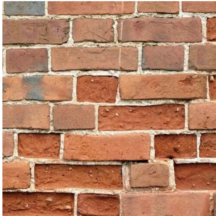
Weathered Brick and Mortar
