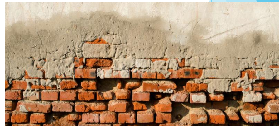
Parging Weathered Brick
